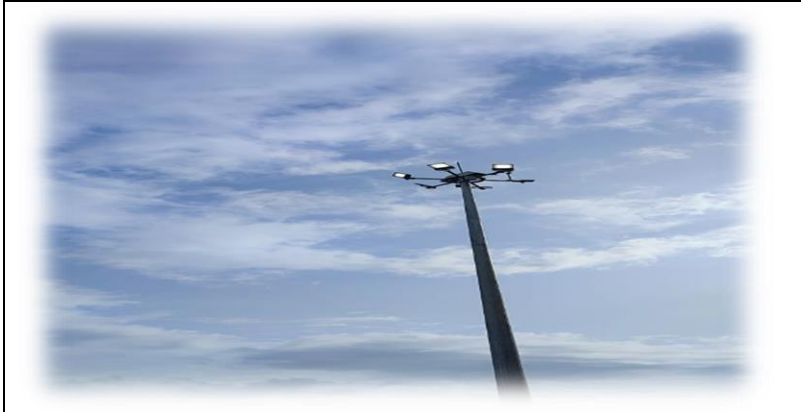
High Mast Poles - Indospace - Chakan - Pune
