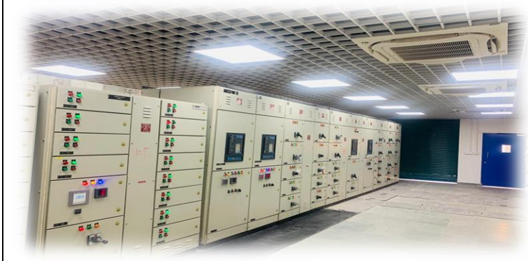
LT Panel Room - M/s. Mastek Ltd. - Mahape - Navi Mumbai.
